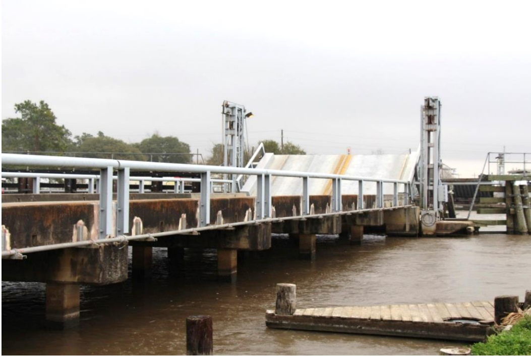
Condition Photo 4: Discoloration from water staining on substructure and curb and condition of steel railing (west approach spans shown).
