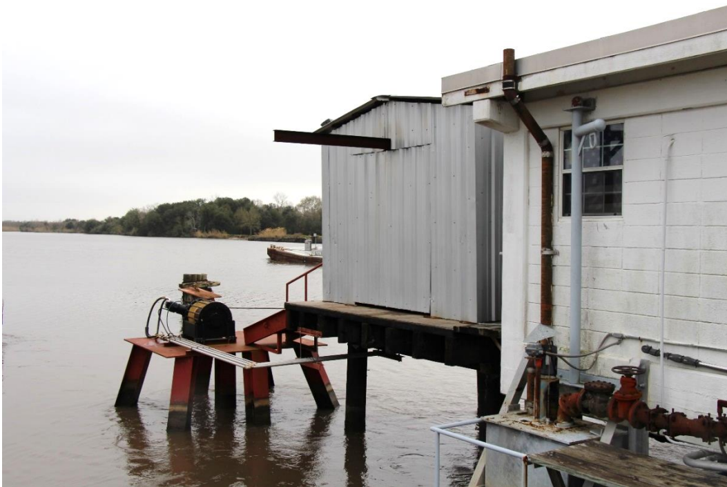
Condition Photo 11: Operator's house and hydraulic equipment shed exterior condition. Also note hydraulically operated winch mounted on pile supported platform.
