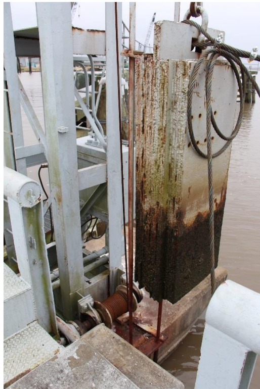
Condition Photo 5: Condition of approach apron lift tower. Rust, corrosion, and section loss on counterweight and counterweight guide bars typical for four counterweights.
