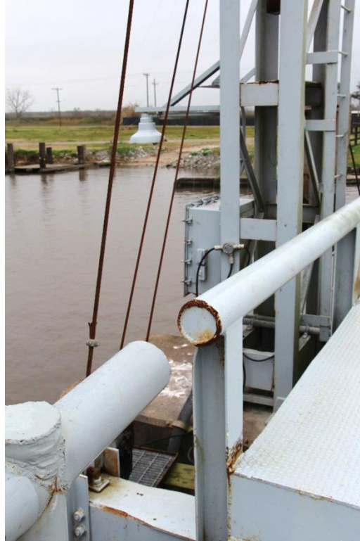
Condition Photo 8: Localized paint failure on steel pipe railing, typical throughout the bridge.
