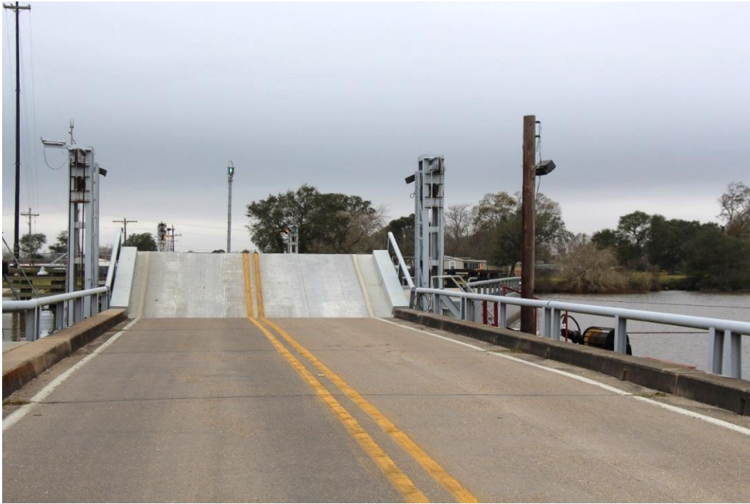
Condition Photo 2: Typical approach apron lift span showing steel plate rotated vertically.
