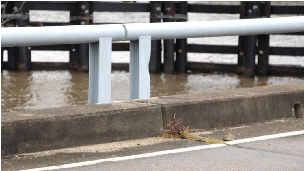
Condition Photo 6: Debris and vegetation on bridge deck, typical on approach spans. Photo also shows condition of railing.
