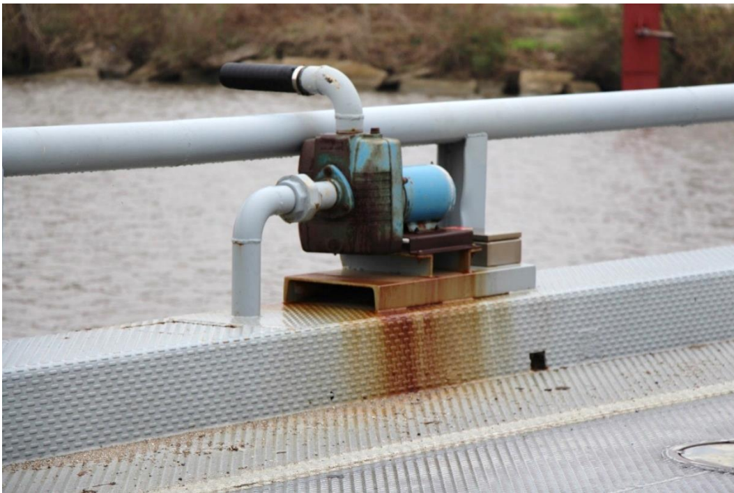
Condition Photo 7: Pontoon pump, one on each corner of pontoon span. The surface rust on the leveling pump and platform is typical for all four pumps.
