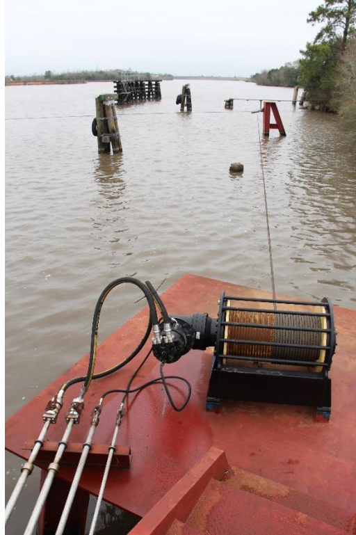
Condition Photo 14: Operating machinery, hydraulically operated winch and cable system, including foundation supports. Note: the winch has been replaced with a system that keeps the cables out of the water.
