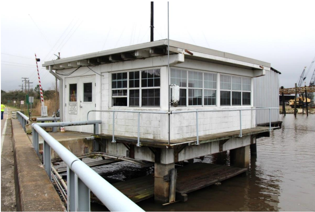
Condition Photo 10: Operator's house exterior condition, with hydraulic equipment shed in background.
