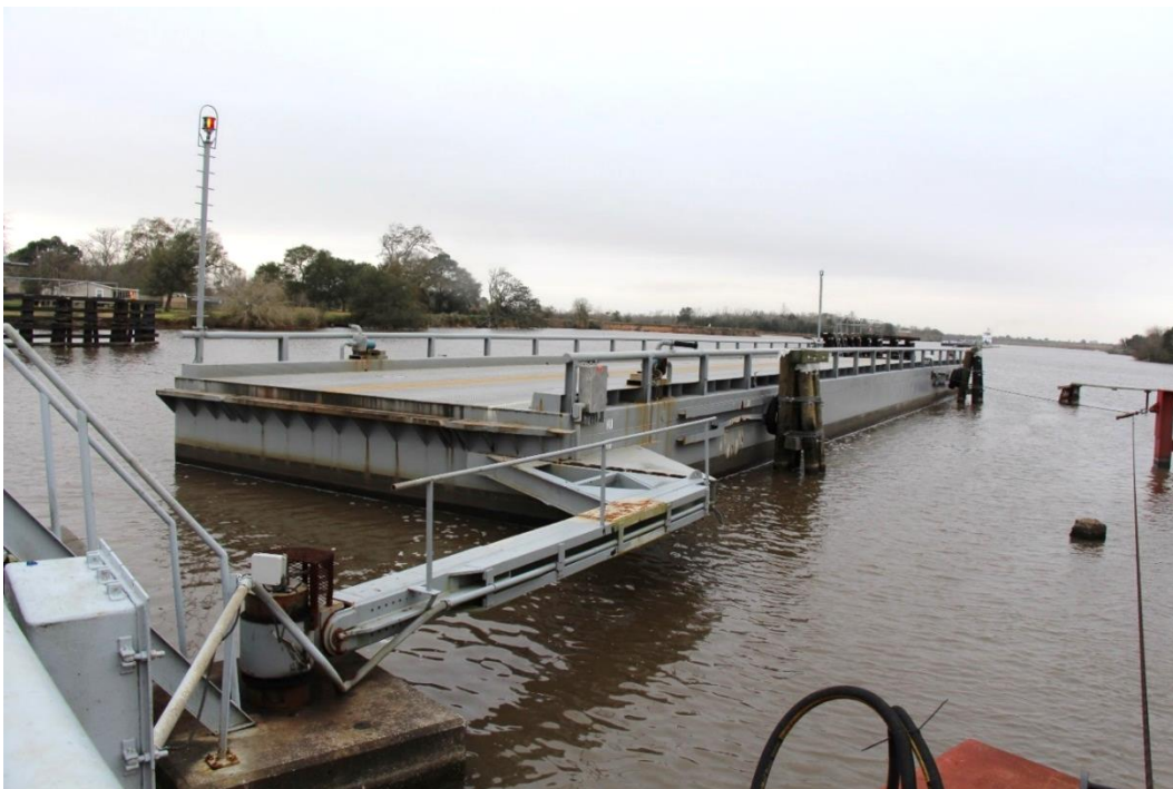
Condition Photo 13: Pontoon swing span in the open position showing pivot arm and support for the pivot arm.
