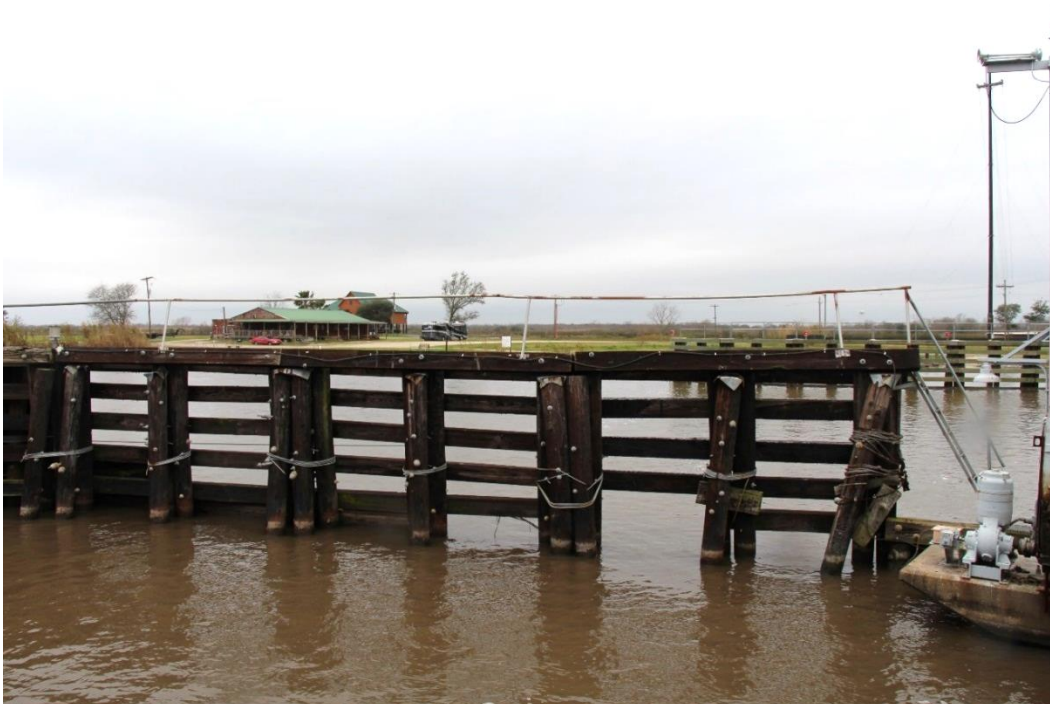
Condition Photo 15: Missing horizontal member and metal railing on southeast timber fender.
