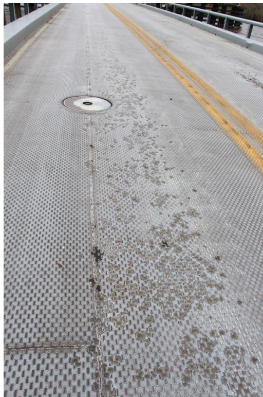
Condition Photo 9: Minor pitting in steel deck on eastbound traffic lane of the pontoon swing span.
