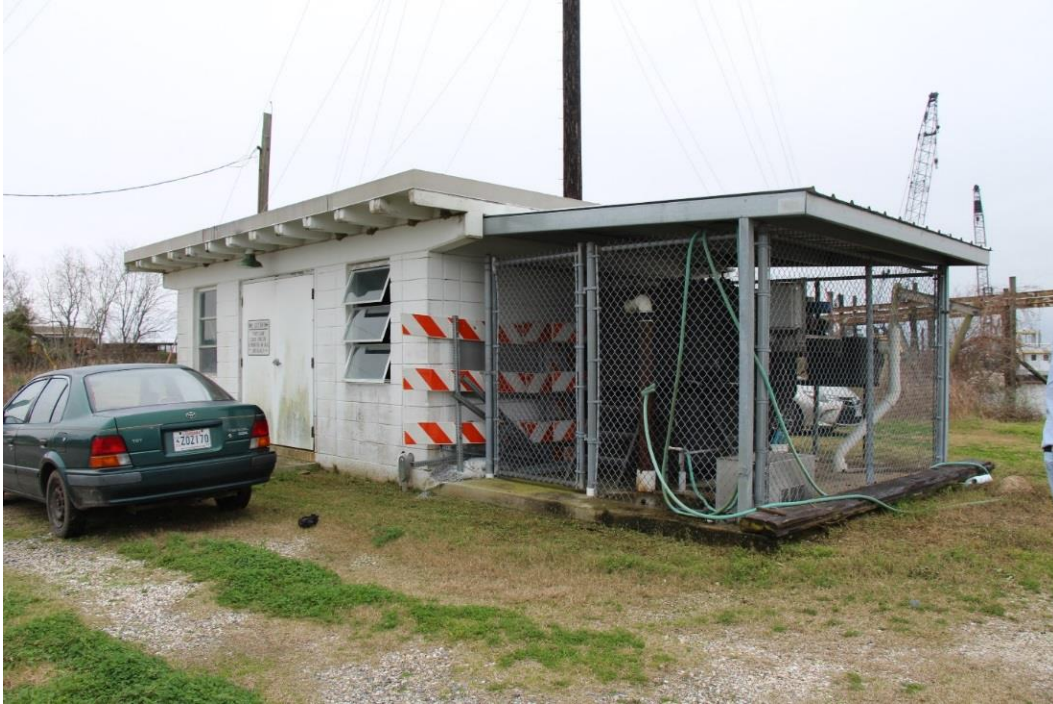
Condition Photo 12: Generator house exterior condition.
